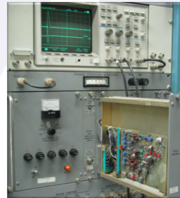
Old analog low-level radio frequency system still in use
